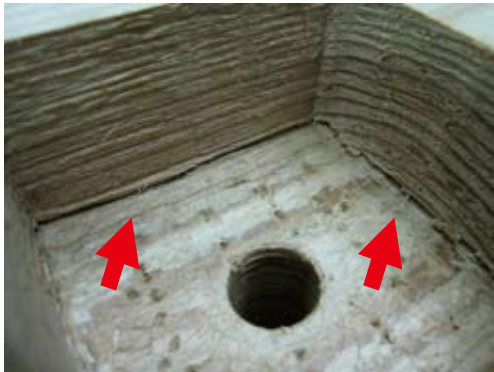
Fig. 5. Wood depression and split at the bottom of the washer notches on the column member.
