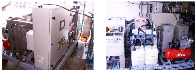
Fig. 2 Photos of the pilot-scale pulsed electrocoagulation treatment system.
