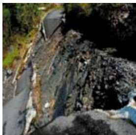
7 K二號橋處嚴重崩塌長度約20 m
