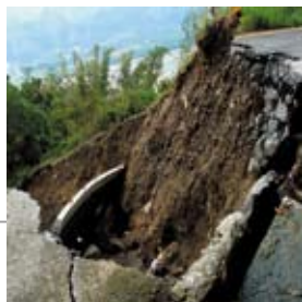
1.7 K路面斷裂深約5 m
