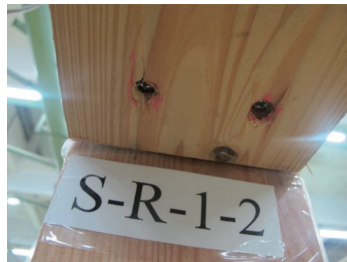
Fig. 9. Screw head depressed at the wood surface after the glulam beam split from the notched corner.
